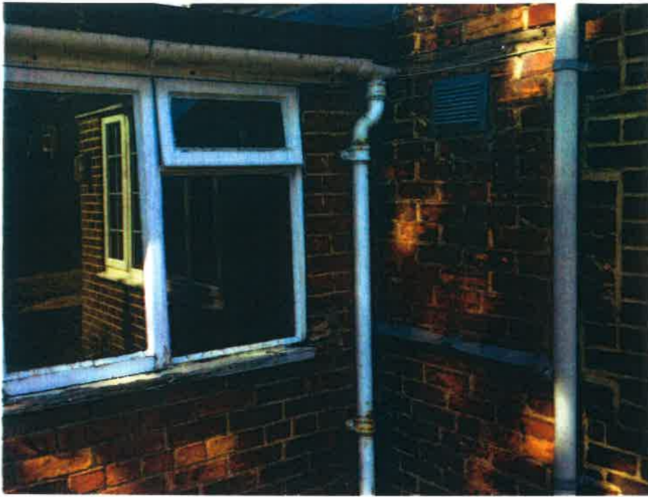
Photograph 19 – West Elevation – lack of vertical DPC between main building and outbuilding add on
