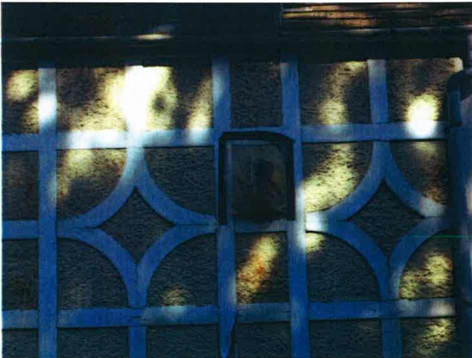
Photograph 18 – West Elevation - Blown render to elevation and high level
