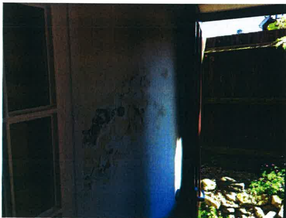
Photograph 10 – Damp staining to internal hallway (shower other side of wall)
