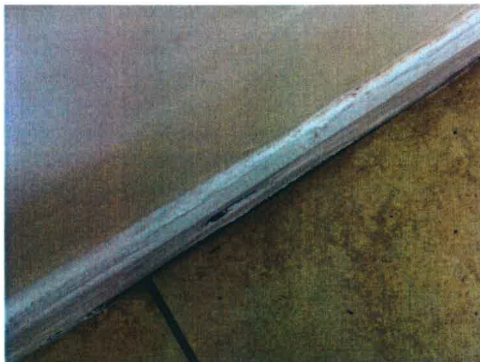
Photograph 12 – Decay to skirting boards in Main Hallway
