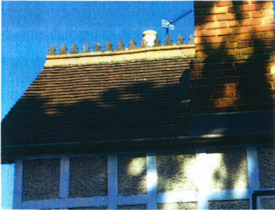
Photograph 17 – West Elevation – slipped / missing tiles and flashing to chimney. Vegetation growth to gutters
