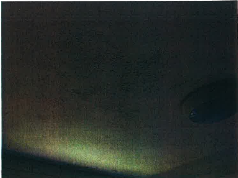
Photograph 14 – Black spot mould to bathroom ceiling
