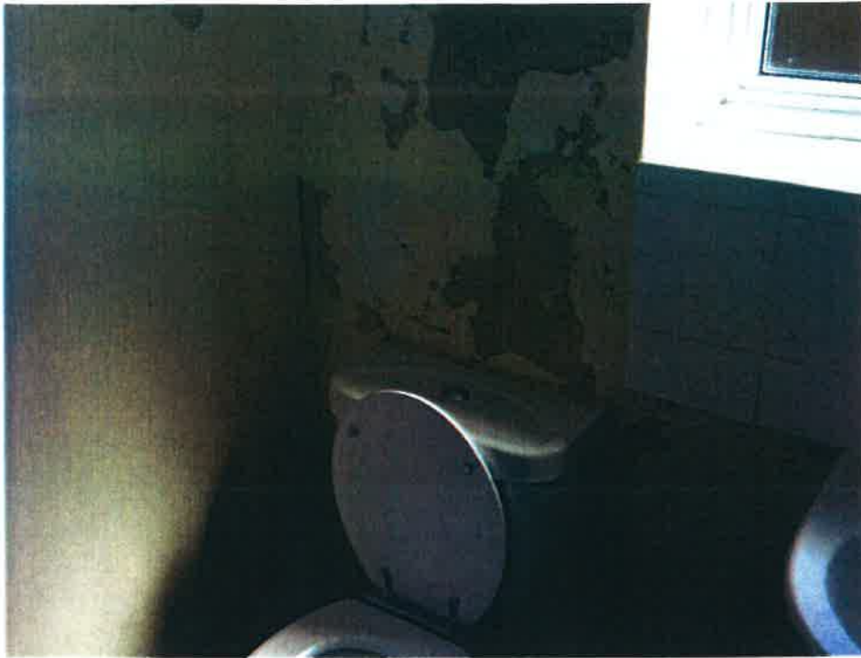
Photograph 15 – Flaking paintwork to bathroom
